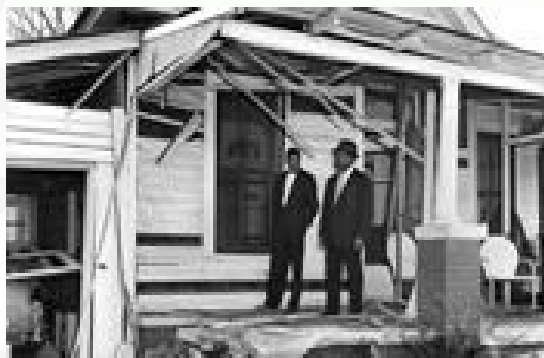
Significant damage to MLK's home
